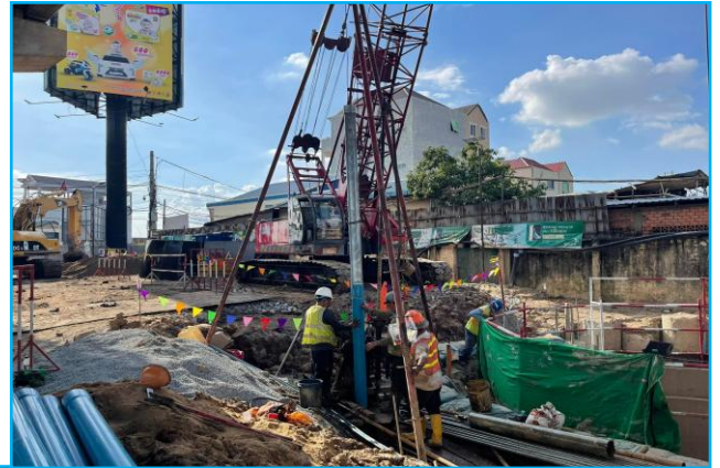
Monitoring groundwater level
